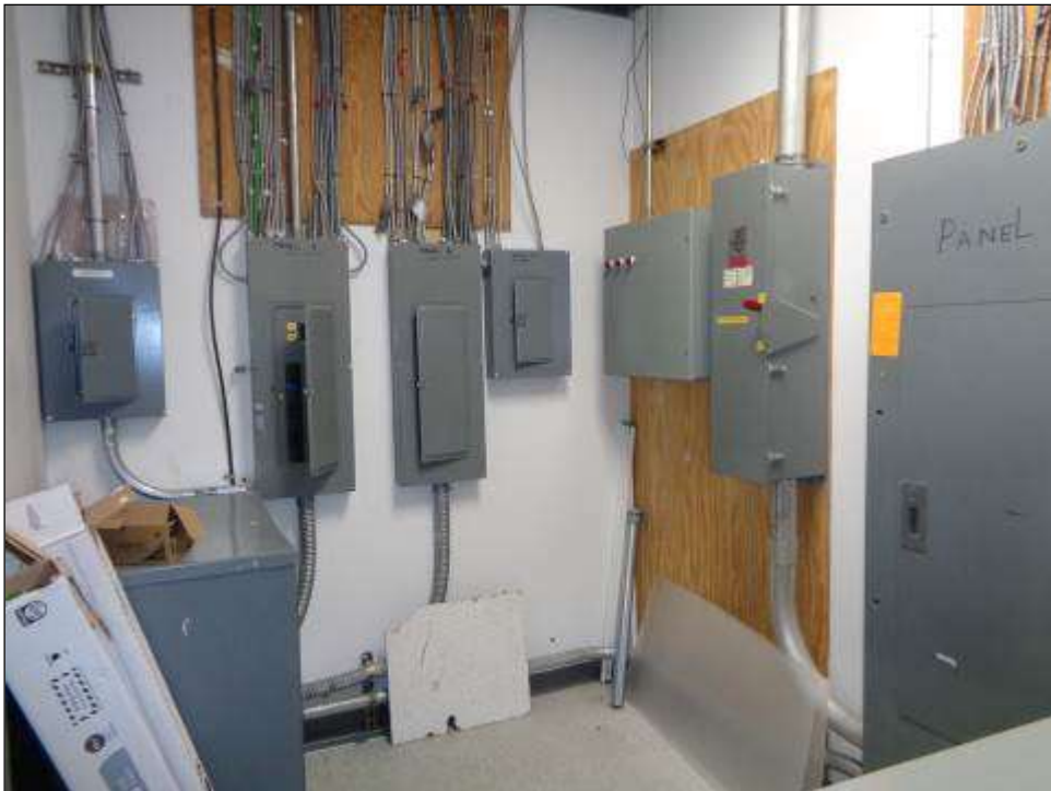
Electrical control room
