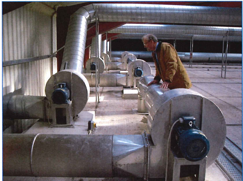
Inspecting components of the aeration system atop a bank of enclosed bays, McGill's most recent process enhancement.
