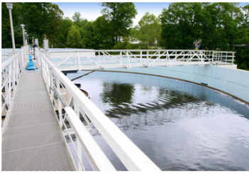
State-of-the-art technology and facilities are hallmarks of Howard County's wastewater treatment.
