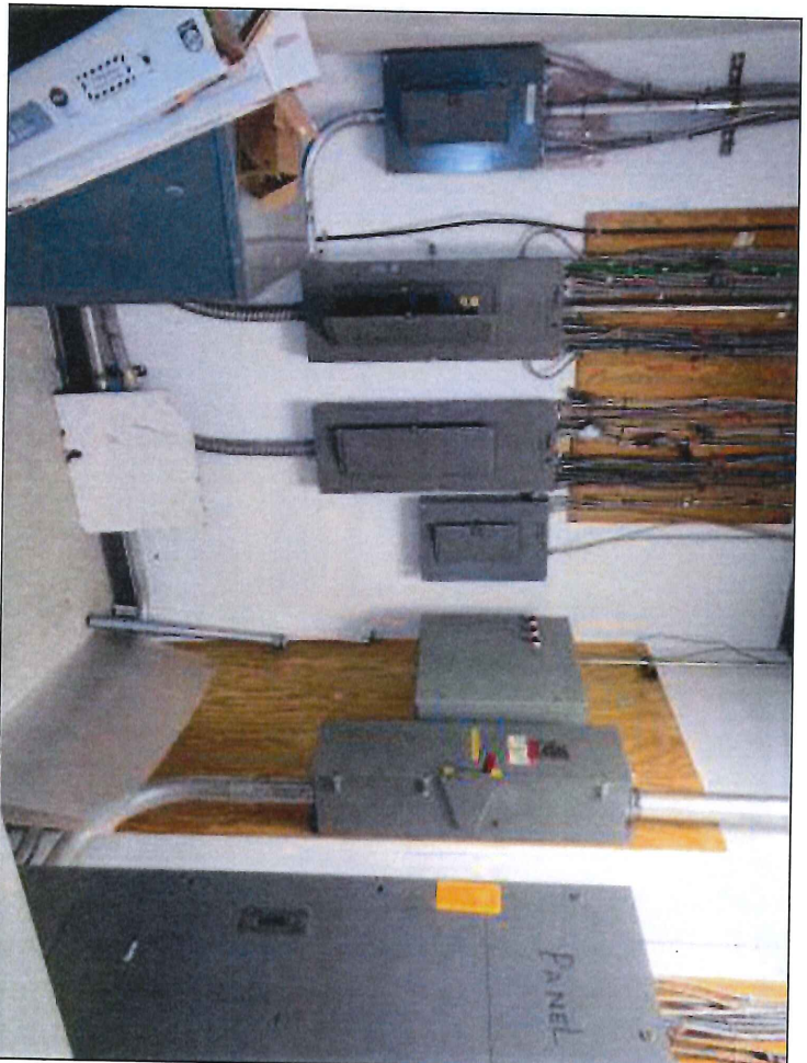
Electrical control room
