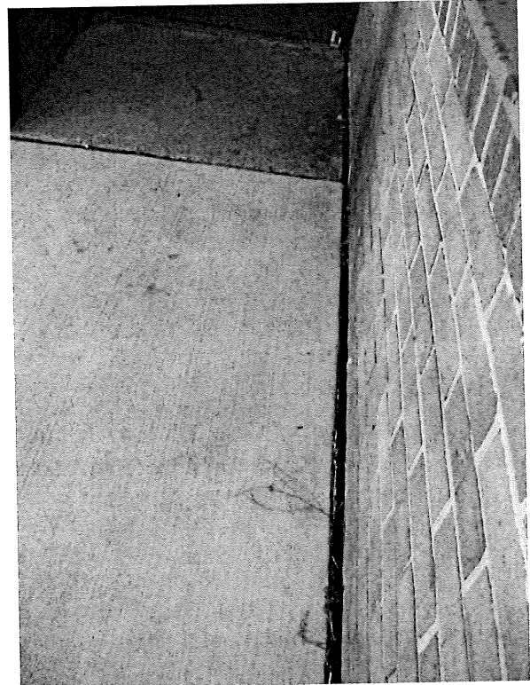
Figure 5 - Missing Caulk Joint
