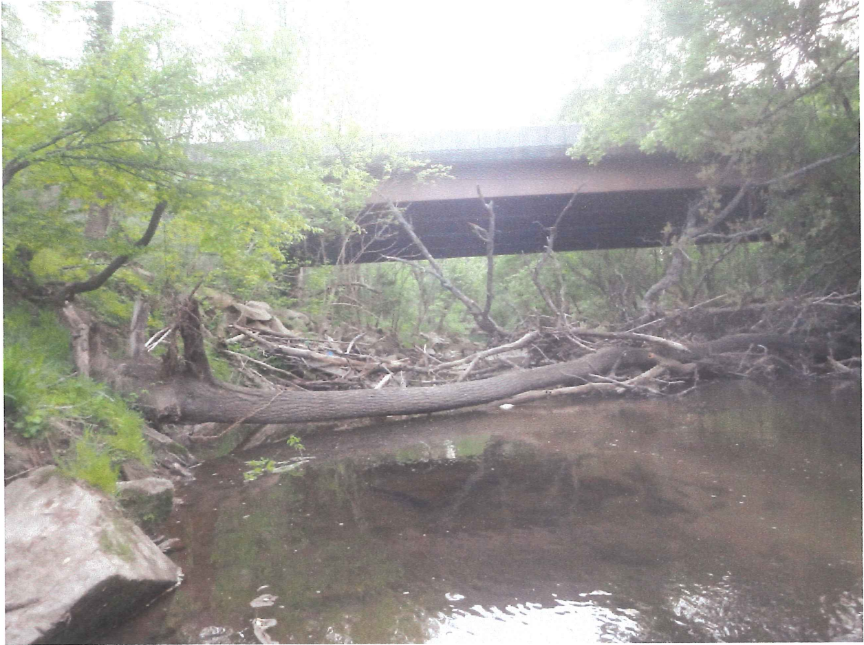
Tree blocking river at Stevens Forrest Road Bridge in 2017
