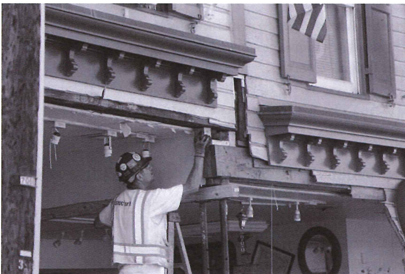
After the 2016 flood, preservation engineers stabilized the interiors of 8111-8113 Main Street. Photo from Patapsco State Heritage Area.
