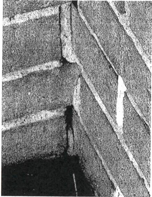
Figure 1 - Brick- Missing Mortar
