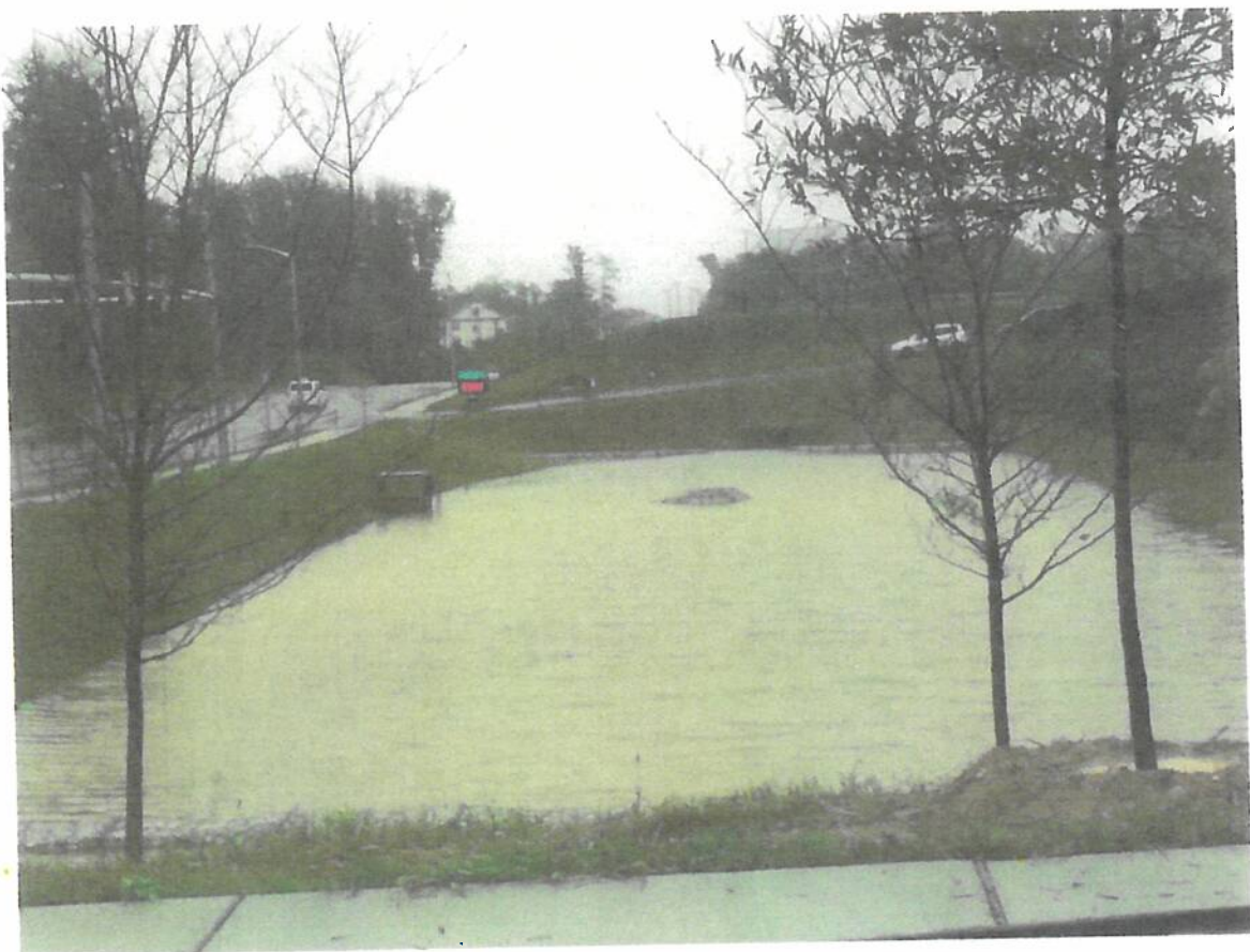
This shows the dry SWM on Lyons Mill road working during a very rainy day
