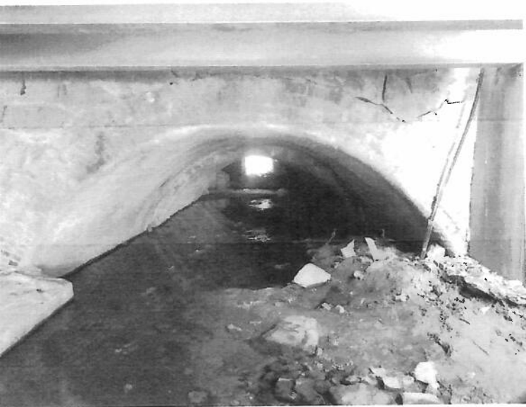
Arched Culvert under main Street Over Three feet of silt and gravel restricting flow
