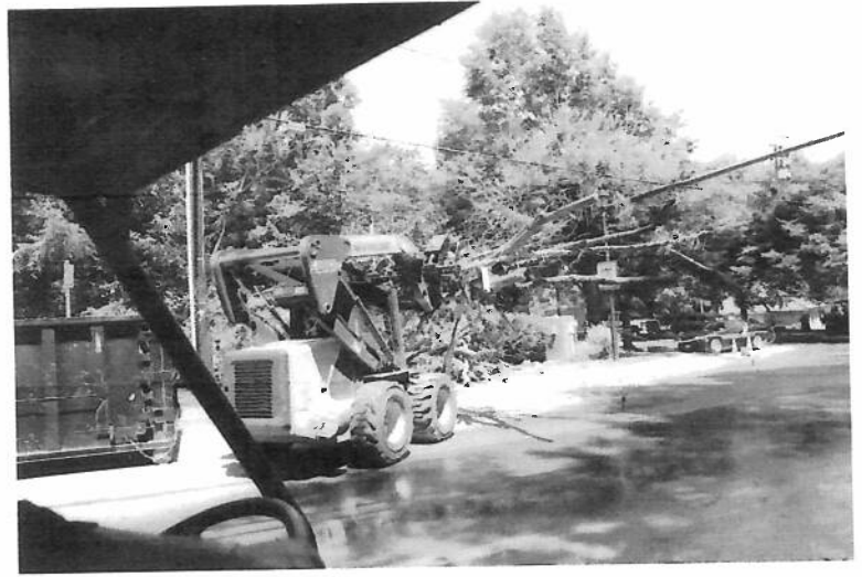
2016 debris clean up at Ellizott Mills
