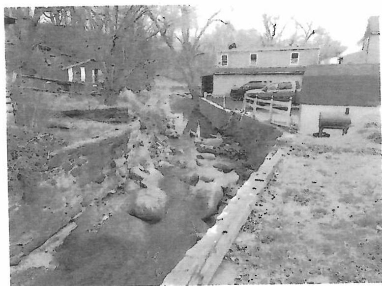
Channel behind Westend houses shows debris that should be removed.
