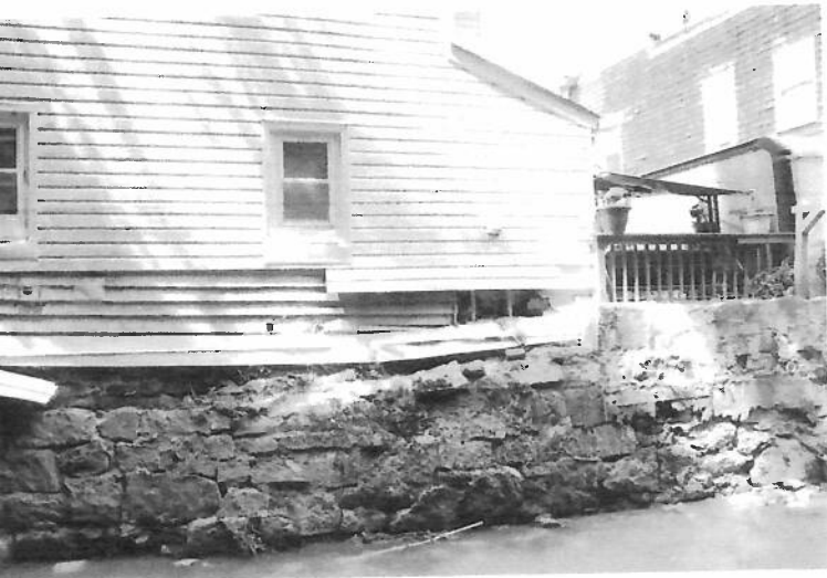
2016 Flood, Floating debris Knocked a hole into the House 8600 Block Westend
