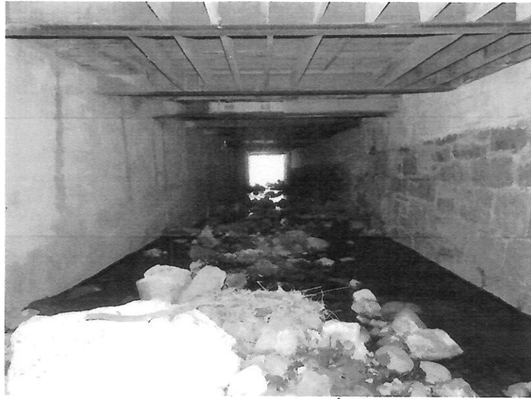
Channel under Lapatupa has tons of debris that needs to be removed
