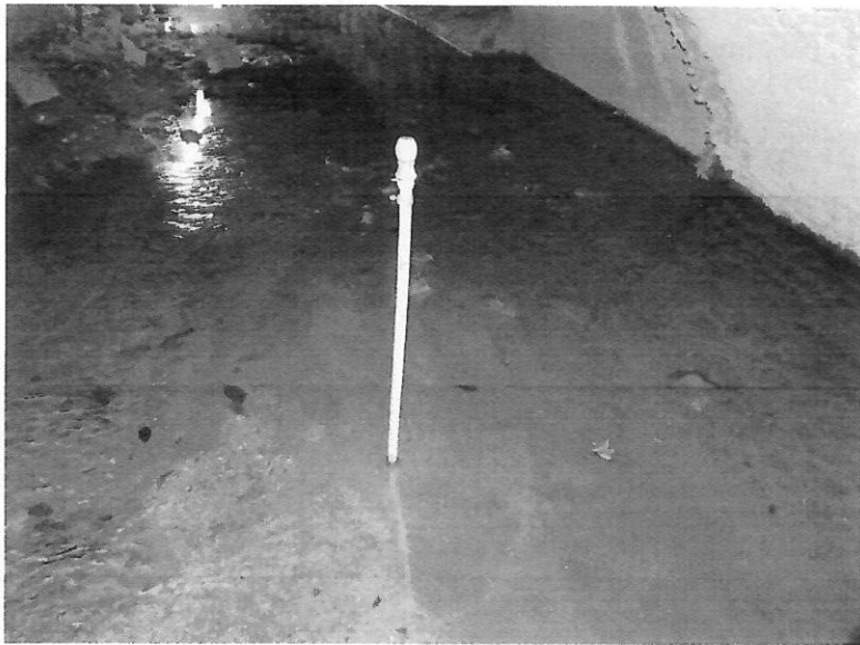
Three feet of sediment under the arched culvert at main street
