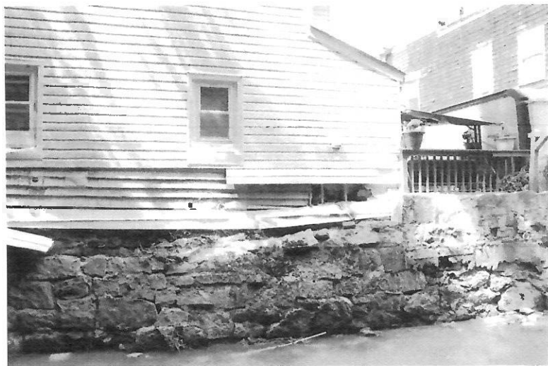
2016 Flood, Floating debris Knocked a hole into the House 8600 Block Westend
