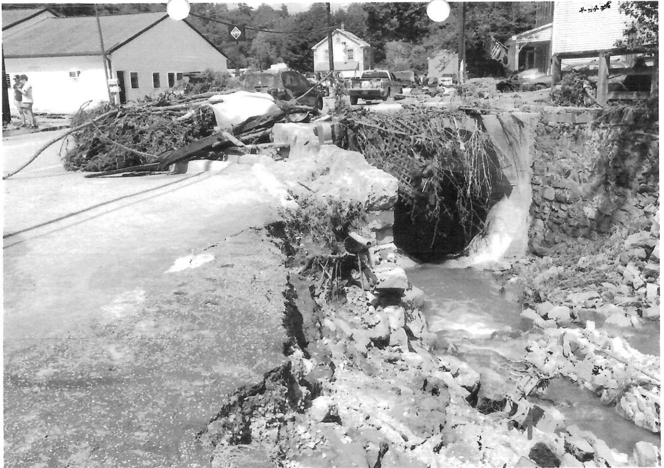
108/84 Culvert, 2016 Flood, Left over debris
