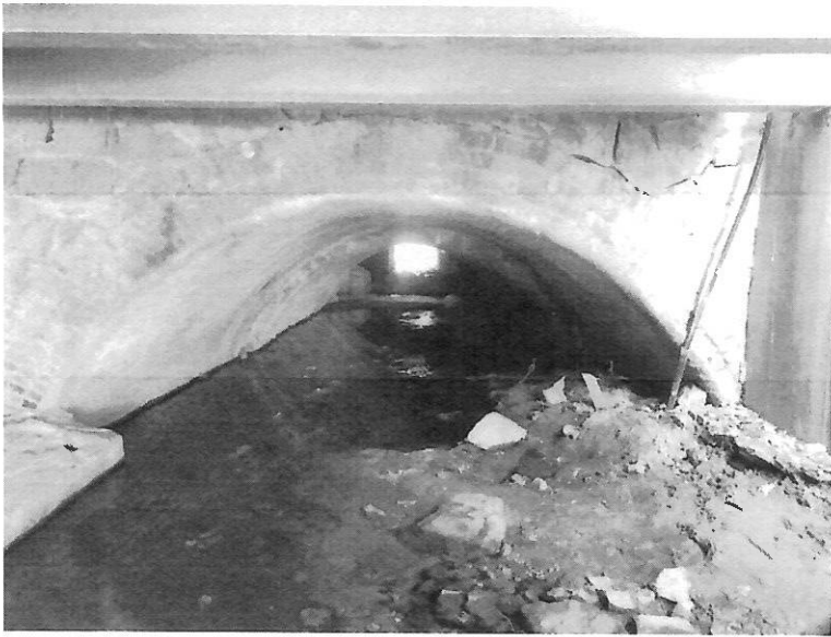
Arched Culvert under main Street Over three feet of silt and gravel restricting flow
