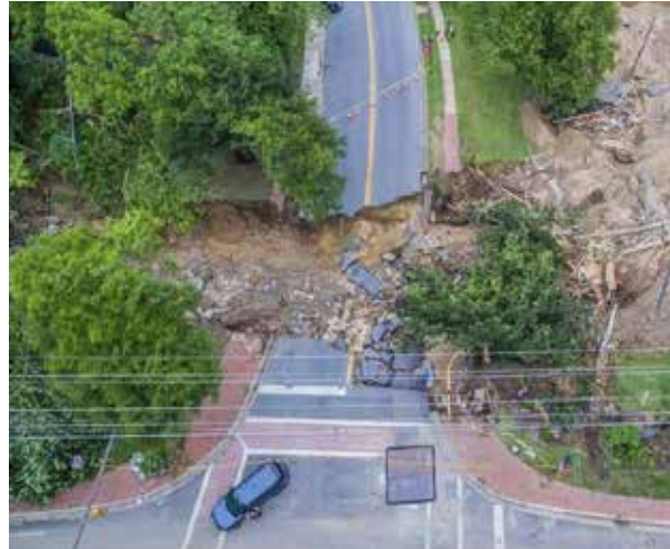
Figure 45: Ellicott Mills Drive Culvert After the 2018 Flood
