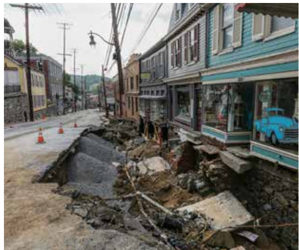
Figure 32: Sidewalk and Utility Damage at 8247 Main Street Immediately Following the 2016 Flood
