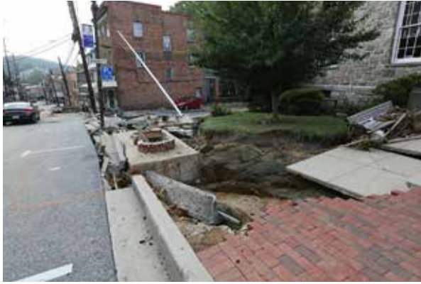
Figure 95: Damage to Brick Paving after the 2018 Flood
