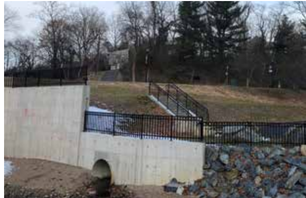
Figure 46: Existing Culverted Stream Outfall in Lot F After the Reconstruction Following the 2018 Flood
