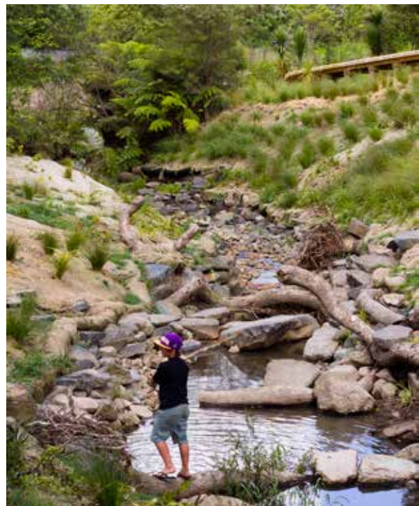
Figure 192: “Green Cultural Trail,” Naturalized Stream Channel Restoration, La Rosa Reserve in New Zealand, Credit: Boffa Miskell, Photographer: Claire Hamilton
