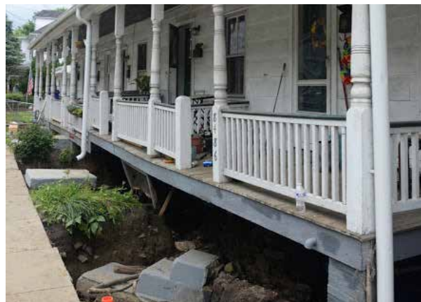
Figure 201: Foundations Scoured by Floodwaters in the West End
