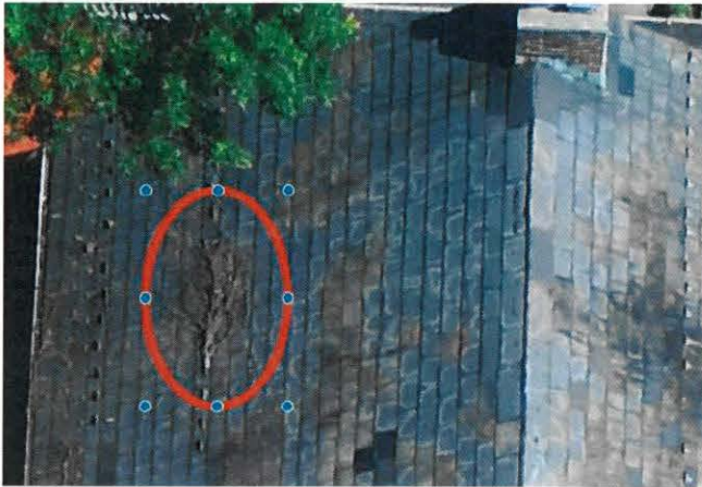
Figure 11 - Aerial view of roof damage.
