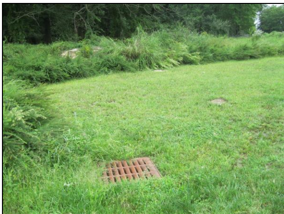
3. View of storm water drain located at the south end of the subject site
