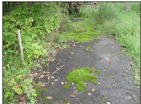
17. View of asphalt-paved walkway located at the east/central area of the subject site
