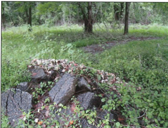
8. View of broken asphalt and walkway at the north/central area of the subject site
