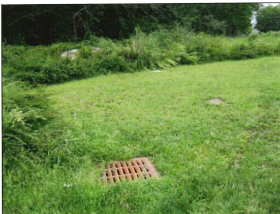
3. View of storm water drain located at the south end of the subject site
