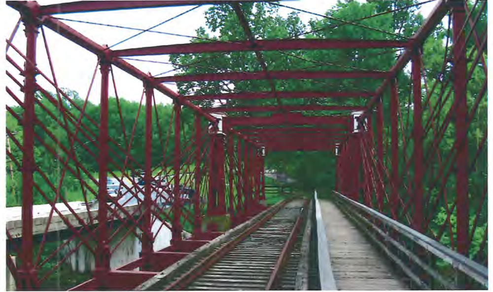
Figure 4.7 Bollman Truss Bridge is one of the two National Historic Landmarks owned by the Department of Recreation and Parks.
