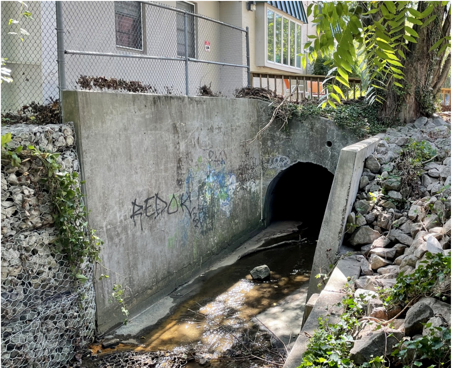
Retaining wall and tunnel at Wyndhurst Avenue that repeatedly floods during periods of heavy rainfall. BELOW: Boulders, some sunken, others pushed together, from a pri
