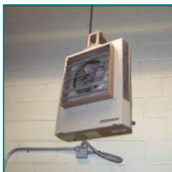
Shop Unit Heater
