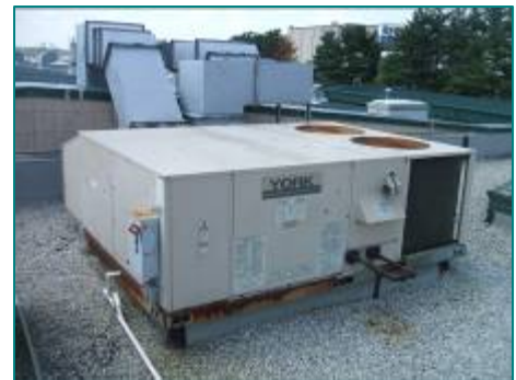
Existing Rooftop Air Handler
