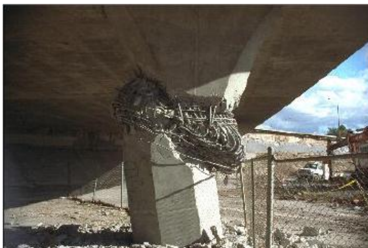
Figure A-12 Earthquake Damage (Source: FEMA)
