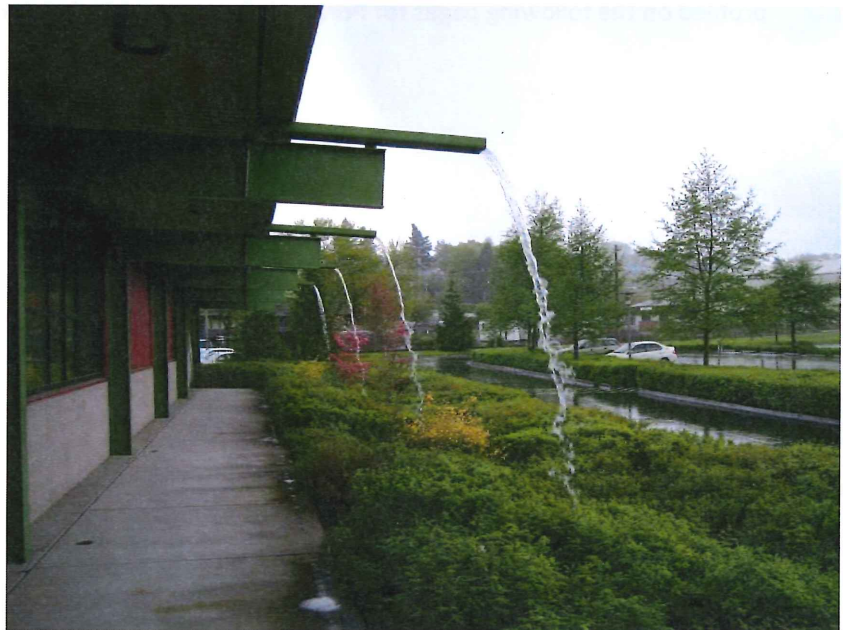
Figure 5. Downspouts at the BES lab disconnected from the combined sewer system and directed into infiltration swales next to the Willamette River (Printed with permission ©2013 Environmental Services, City of Portland, OR)
