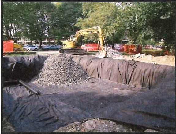
Figure 14: Stormwater trench at Columbus Square.
