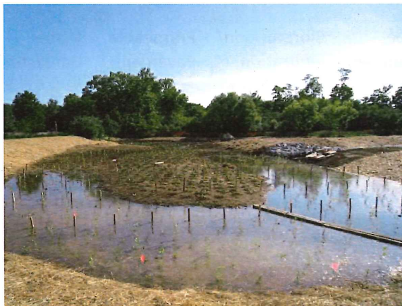
Anne Arundel County has identified 455 stormwater ponds that are slated to be retrofitted to provide water quality treatment, such as in this photo (Source: Center for Watershed Protection)
